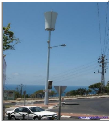
Figure 2: Small Wireless Support Structure
